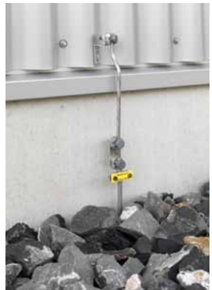
Separation point in an earthing system
