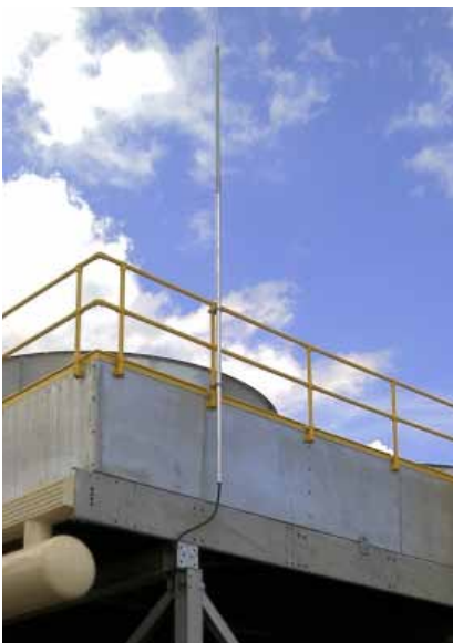
Insulated arrestor system in an explosion-prone area
