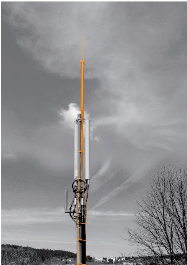
Cell tower with isCon® conductor
