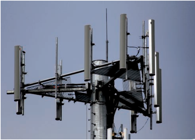
Mobile telecommunications mast
