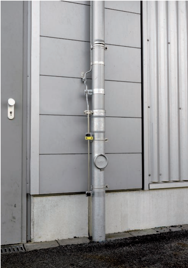
Lightning down-conductor at a downpipe
