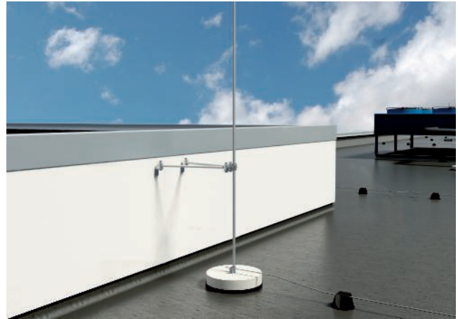
Isolated lightning protection with insulating beams
